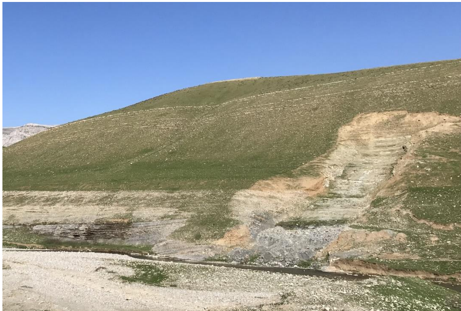
The first attempt at constructing the Chaq Chaq 2 Dam was unsuccessful; it was found that the rock slopes were unstable. The scars in the rocks are still visible. (2020)
