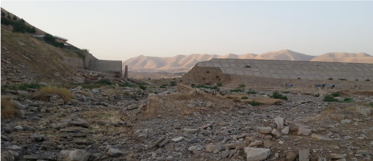
The Chaq Chaq Dam collapsed in 2006. (2016)
